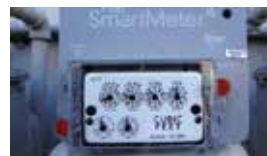
Automated Meter Reading
