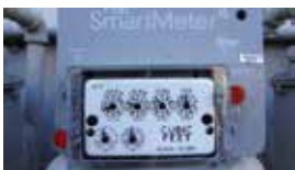
Automated Meter Reading
